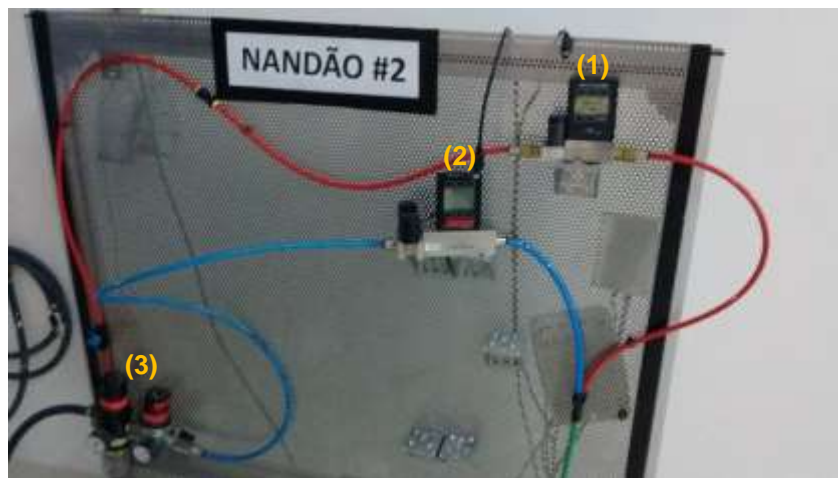
Figure 5 – Flow meters installation: (1) methane stream ( Q_{max} = 5 SLPM), (2) air stream ( Q_{max} = 50 SLPM) and (3) pressure gauge and air filter regulator.
